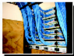
LAN & WAN Installation
